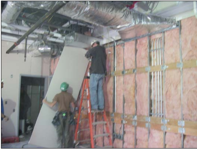
Photo 11 (1417): Shows Dirago Drywall Co. crew installing sheet rock in the training room.
