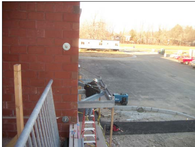
Photo 24 (1485) : Shows Davis Erectors Co. crew welding on the canopy over the exterior stairway door.
