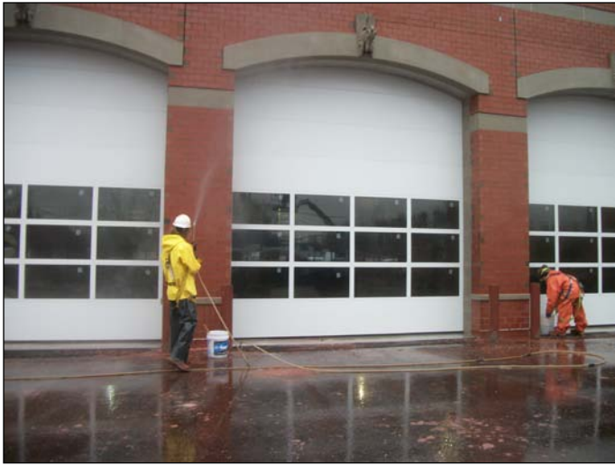
Photo 3 (1396) : Shows Nate Libby Masonry Construction Co. crew power washing the brick veneer of the fire station building.
