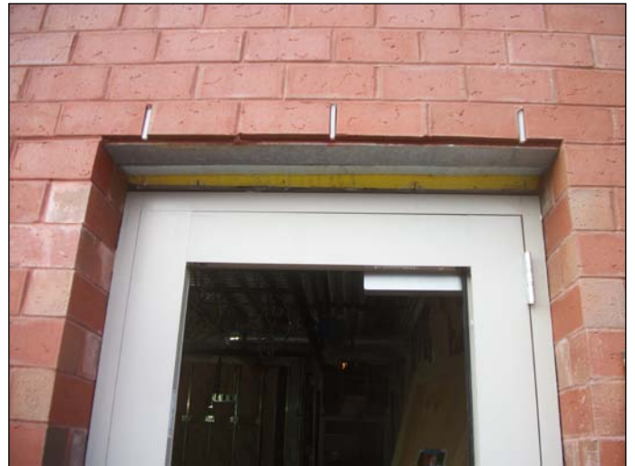
Photo 14 (1423): Shows Glass Pro Co. crew installed the aluminum door to the training room.
