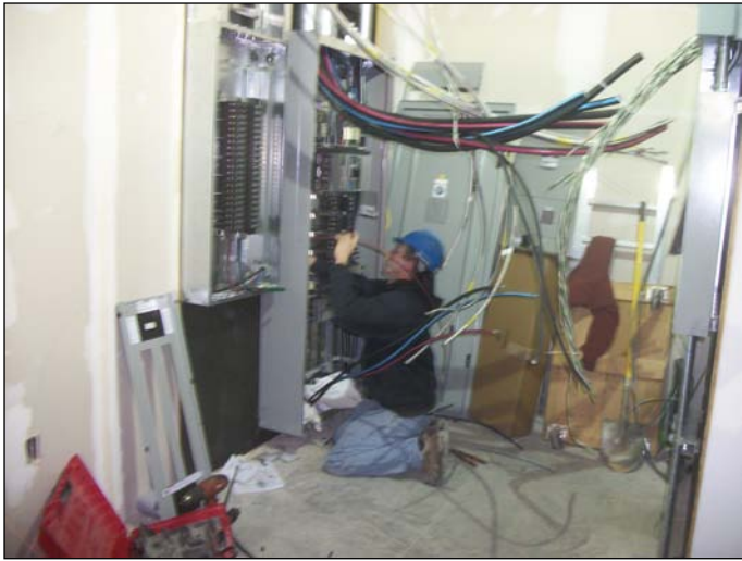
Photo 15 (1436): Shows BH Milliken Electrical Co. crew terminating wires in a panel in the electrical room.
