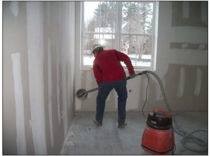
Photo 16 (1442): Shows Dirago Drywall Co. crew sanding the mudded joints in the first floor Administration area.
