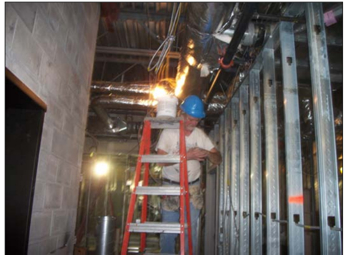
Photo 6 (1399) : Shows Maine Tech Air sealing duct work in the first floor Administration area.
