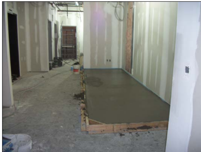
Photo 20 (1461) : Shows Pizzagalli Corp. Co. crew placed concrete in the pad for the fire wagon display.
