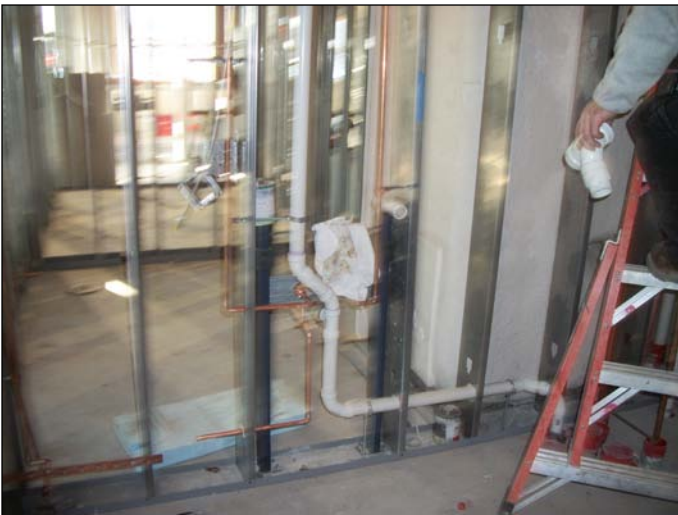
Photo 9 (1430): Shows Titan Mechanical Co. crew installing vent piping in the second floor Administration area bathrooms.
