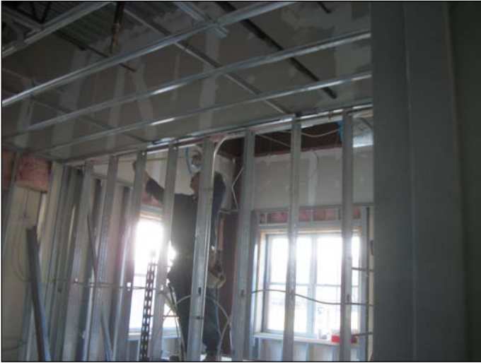
Photo 27 (1472) : Shows SMR Roofing Co. crew set the skylight in the gym on the second floor Administration area.
