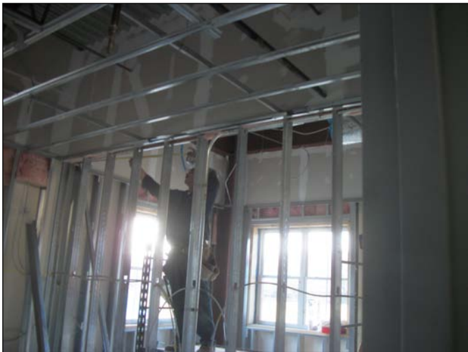
Photo 23 (1472) : Shows Dirago Drywall Co. crew installing framing in the ceilings of the second floor Administration area.
