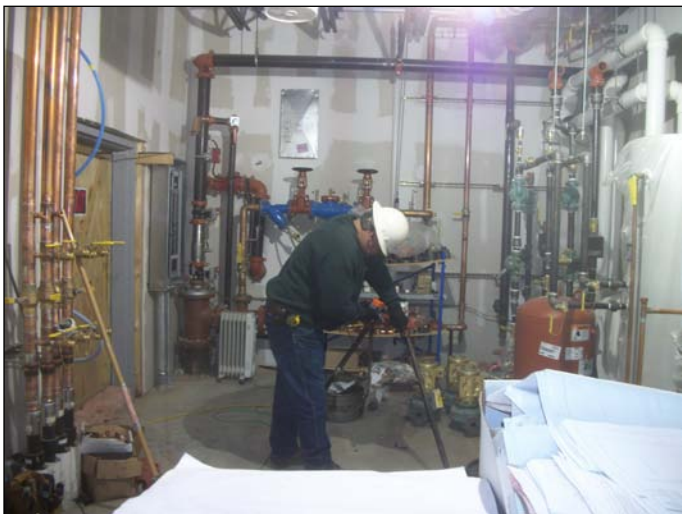
Photo 21 (1466) : Shows Titan Mechanical Co. crew installing mechanical piping and equipment in the mechanical room.
