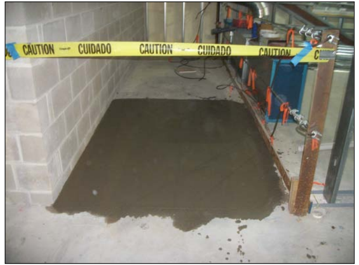
Photo 8 (1401): Shows Pizzagalli Corp. Co. crew placed concrete in an opening in the slab of the day room.
