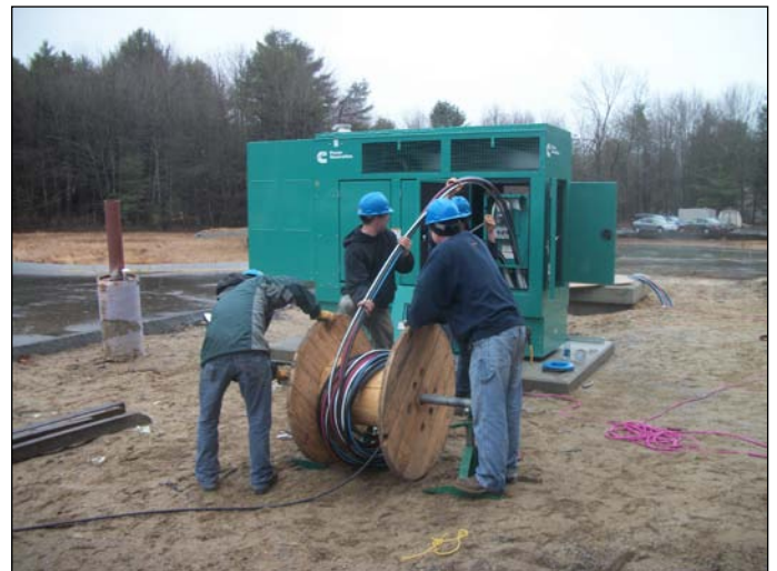
Photo 2 (1387) : Shows BH Milliken Electrical Co. crew pulling wires to the emergency generator, electrical panels, etc.
