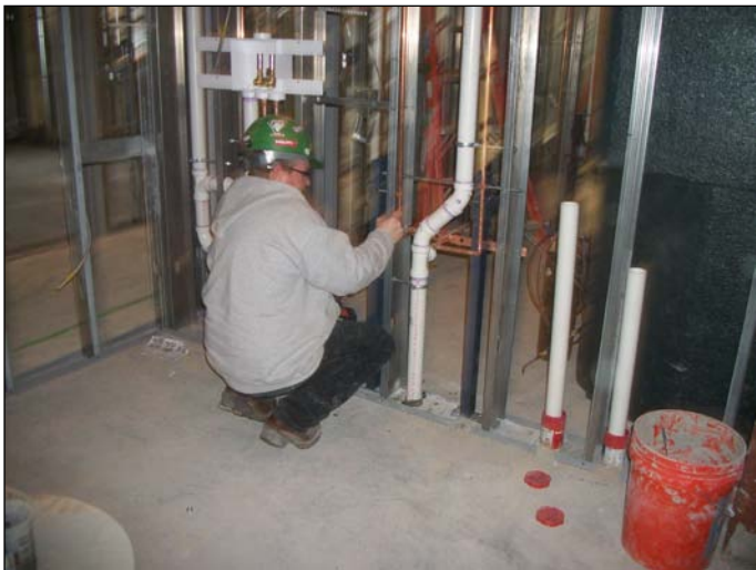
Photo 1 (1400) : Shows Titan Mechanical Co. crew installing hot and cold water piping to the bathrooms in the second floor Administration area.
