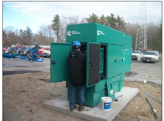
Photo 10 (1422): Shows BH Milliken Electrical Co. crew terminating wires to the emergency generator.
