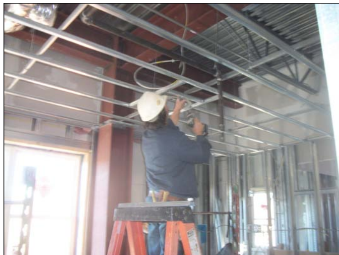
Photo 26 (1498) : Shows Dirago Drywall Co. crew framing ceilings in the second floor Administration area.
