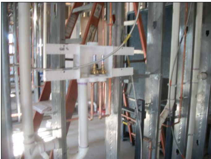
Photo 25 (1499) : Shows Titan Mechanical Co. crew tested the domestic piping in the wall framing. Passed the pressure test.
