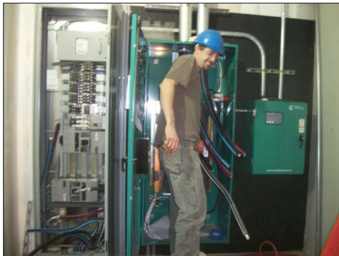
Photo 22 (1469) : Shows BH Milliken Electrical Co. crew terminating wires in the emergency transfer switch panel.
