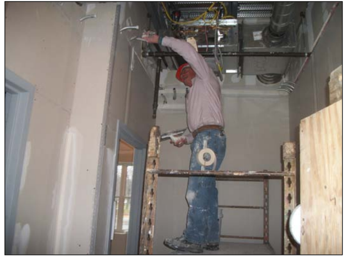
Photo 4 (1395) : Shows Dirago Drywall Co. crew taping and mudding joints in the sheet rock in the first floor Administration area.
