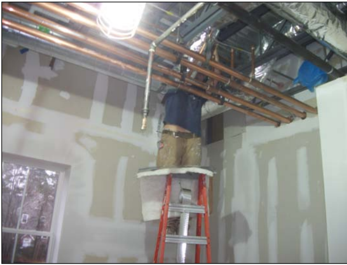
Photo 7 (1392): Shows Hi Tech Insulation Co. crew insulating the duct work in the first floor Administration area.
