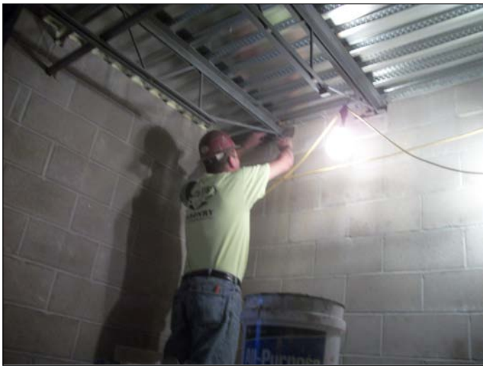
Photo 17 (1448): Shows Nate Libby Masonry Construction Co. crew installing brick in the pockets for structural trusses in the rooms under the Mezzanine.
