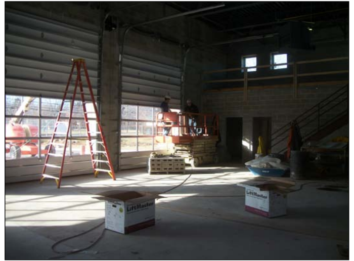
Photo 12 (1416): Shows Overhead Door Co. crew installing weather seals on the overhead door openings.
