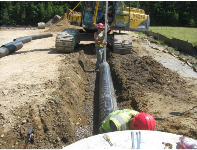
Photo 5 (4525) : Shows Peters Construction Co. crew installing 12" ADS storm drain piping from catch basin No. 7 to catch basin No. 9..
