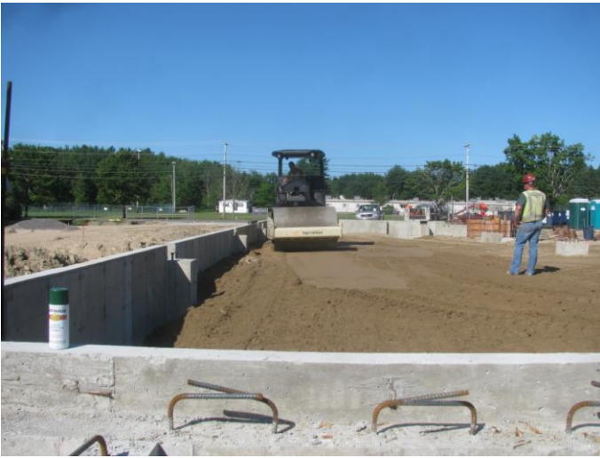
Photo 1 (4497) : Shows Peters Construction Co. crew placing and compacting gravel on subgrade of interior of fire station at "A" line.
