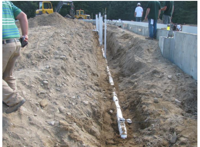
Photo 8 (4536) : Shows Peters Construction Co. crew has excavated for Titon Mechanical Co.'s crew to install sanitary piping under slab of administration area.
