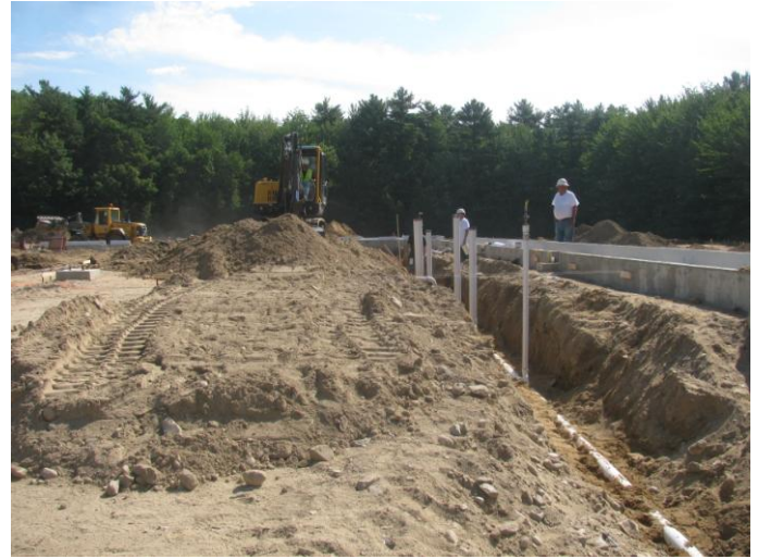
Photo 10 (4539): Shows Titon Mechanical Co. crew has installed sanitary piping in subgrade of administration building area.
