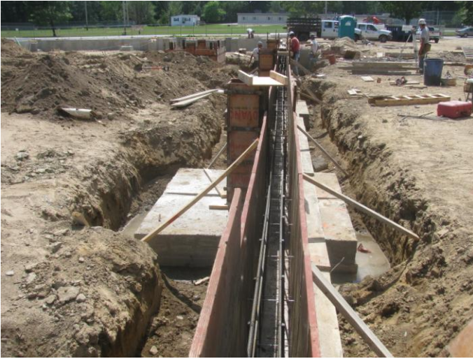
Photo 9 (4544): Shows Lajoie Bros. Construction Co. crew has placed reinforcing steel in wall forms on "C" line of building.
