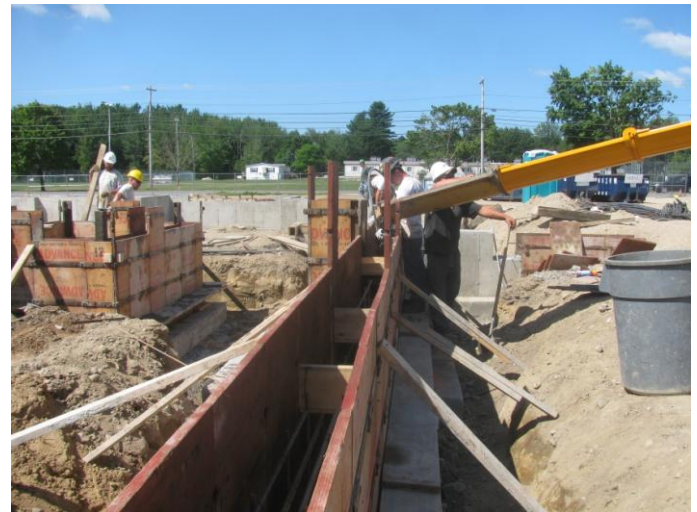
Photo 12 (4556): Shows Lajoie Bros. Construction Co. crew placing concrete in wall forms on "C" line.
