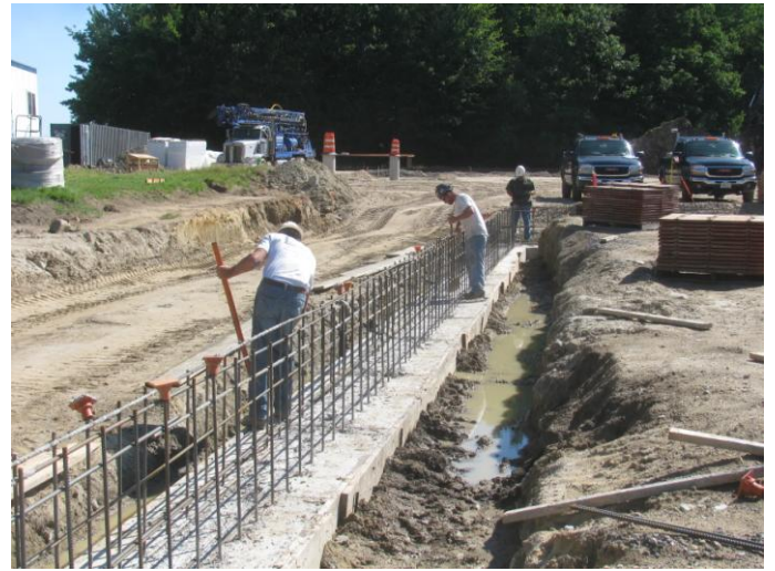
Photo 2 (4502) : Shows Lajoie Bros. Construction Co. crew installing reinforcing steel in wall on north side of Central Fire Station.
