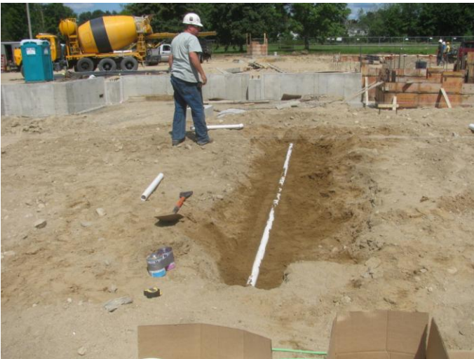
Photo 11 (4560): Shows Peters Construction Co. crew has excavated for sanitary piping below first floor slab of administration area.
