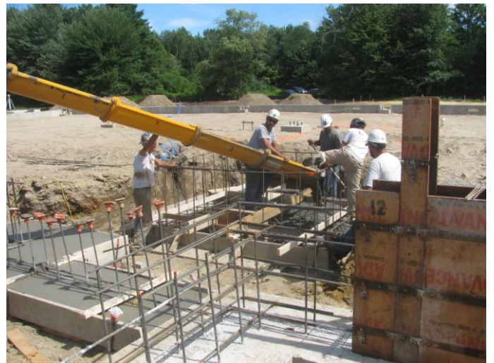
Photo 4 (4515) : Shows Lajoie Bros. Construction Co. crew placing concrete in central wall footing and elevator sump footing.
