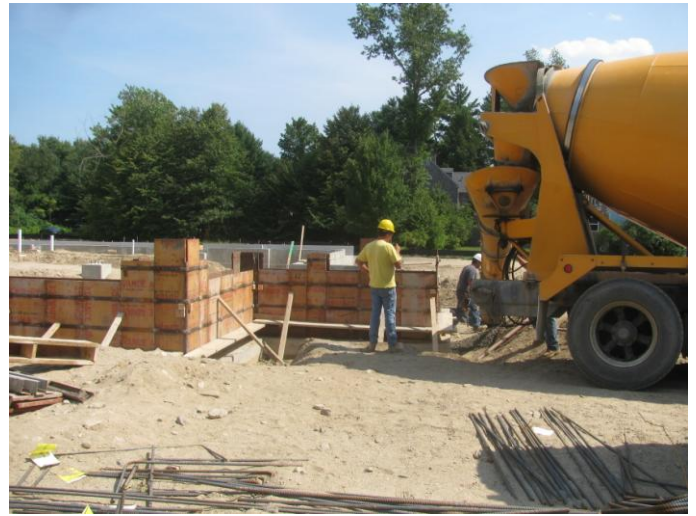
Photo 6 (4527) : Shows Lajoie Bros. Construction Co. crew placing concrete in wall forms west wall of Central Fire Station.
