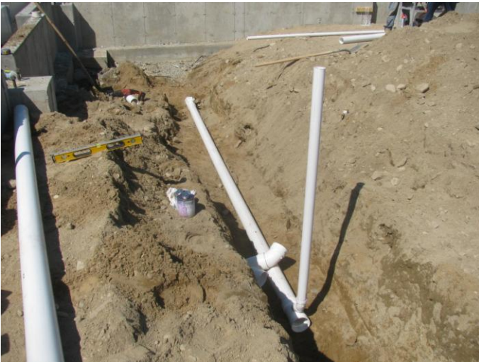
Photo 7 (4523) : Shows Titon Mechanical Co. crew has installed 4" PVC sanitary piping under slab, first floor of administration area of Central Fire Station.
