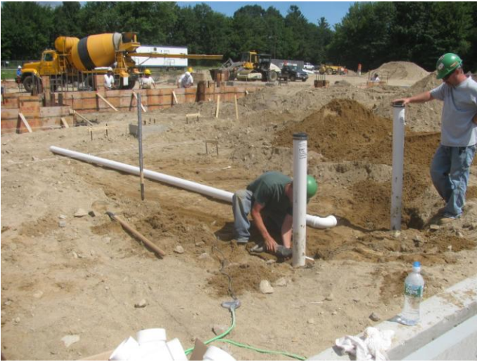
Photo 13 (4561): Shows Titon Mechanical Co. crew installing sanitary piping under first floor slab of administration area.
