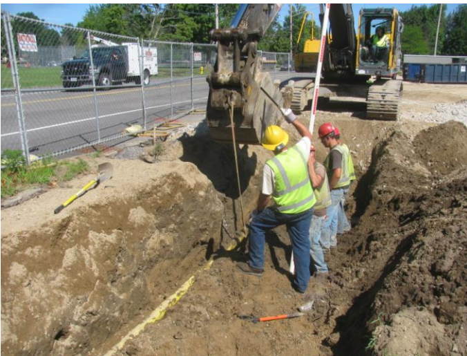
Photo 3 (4508) : Shows Peters Construction Co. crew raising existing 4" PPE gas main piping along North Street.
