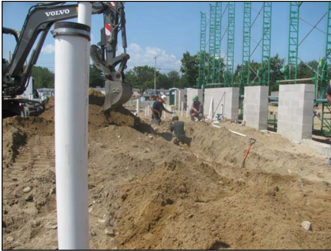
Photo 21 (4659): Shows Nate Libby Masonry Construction Co. crew working on east wall of the Apparatus Bay.
