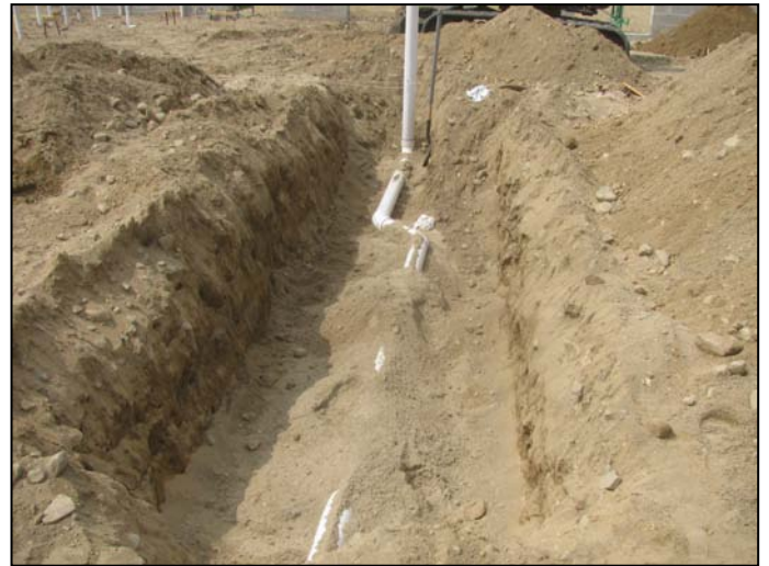
Photo 16 (4643): Shows Titon Mechanical Co. crew installing sanitary piping in subgrade at the southeast corner of the Administration area.
