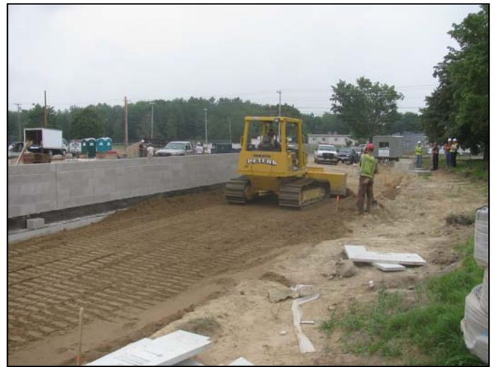
Photo 14 (4634): Shows Peters Construction Co. crew placing gravel and compacting material in the rear parking lot.
