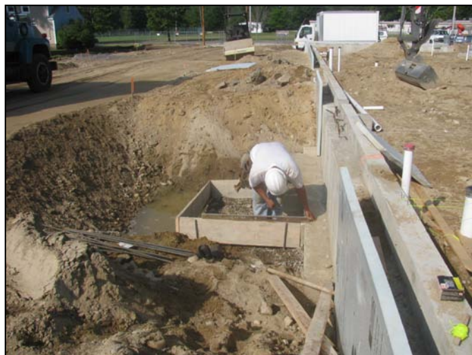
Photo 19 (4655): Shows Lajoie Bros. Construction Co. crew installing foundation footing forms for the south side door entrance.
