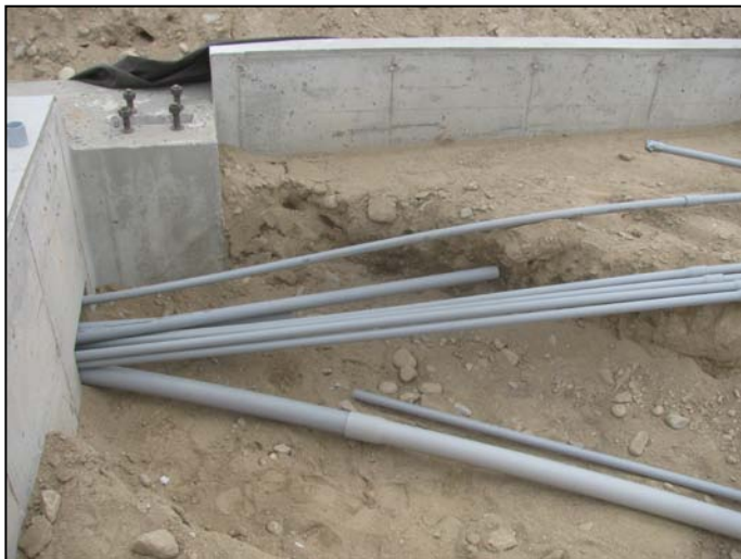
Photo 17 (4640): Shows BH Millekin Electrical Co. crew installing PVC conduit to the interior of the fire station.
