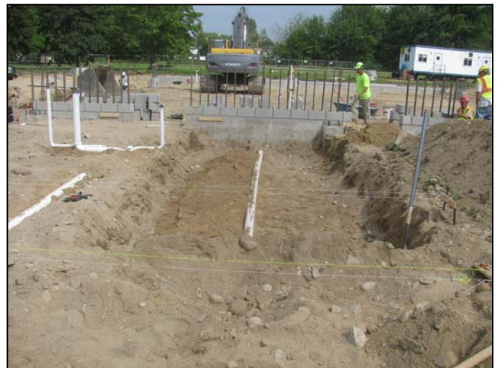
Photo 8 (4594) : Shows Titon Mechanical Co. crew installing sanitary piping in subgrade of Administration area.
