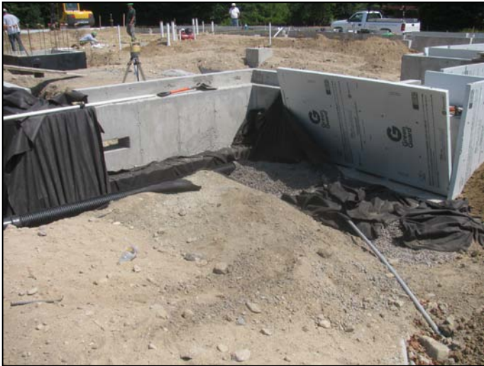
Photo 1 (4573): Shows Peters Construction Co. crew placed gravel and compacted interior of west wall by entrance to fire station.
