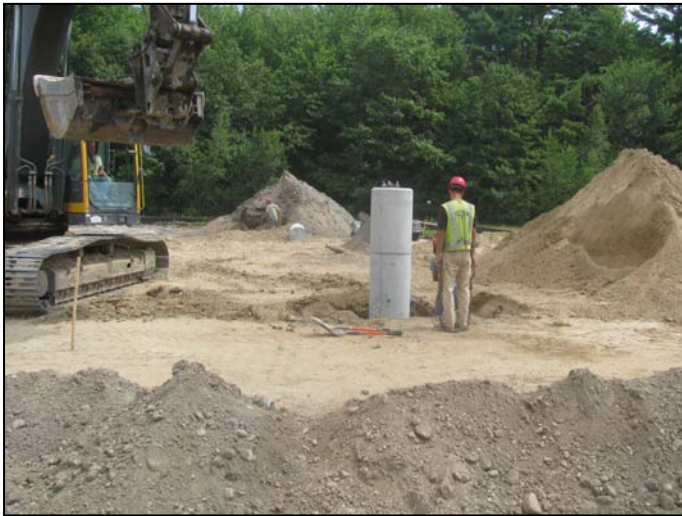
Photo 5 (4596) : Shows Peters Construction Co. crew installing light pole base in rear parking lot.
