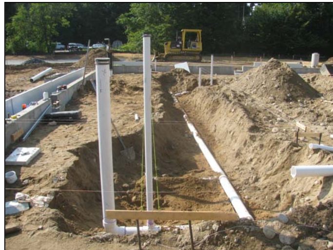
Photo 20 (4654): Shows Titon Mechanical Co. crew installing sanitary piping in subgrade near the "6" line and "C" line of the building.
