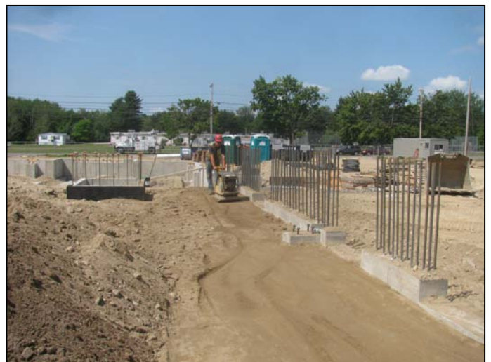
Photo 4 (4570): Shows Nate Libby Masonry Co. crew placed concrete masonry block on north and west wall of the Apparatus building.
