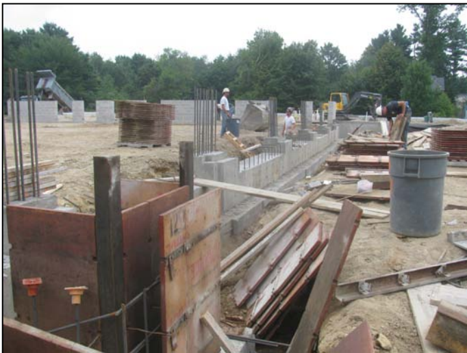
Photo 15 (4632): Shows Lajoie Bros. Construction Co. crew installing forms and reinforcing steel for west wall of the Apparatus Bay.
