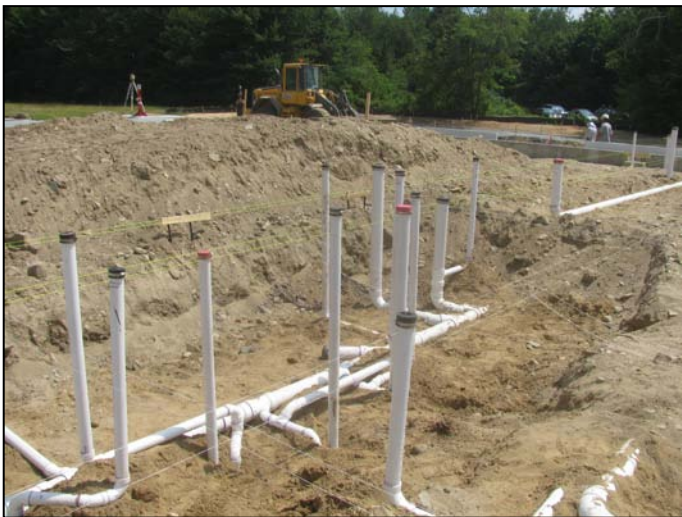
Photo 11 (4618) : Shows Titon Mechanical Co. crew installing sanitary piping in subgrade of Administration area of the fire station.
