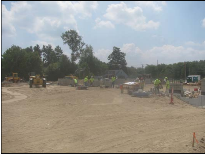
Photo 9 (4611) : Shows Peters Construction Co. crew placing and compacting gravel in the rear parking lot.
