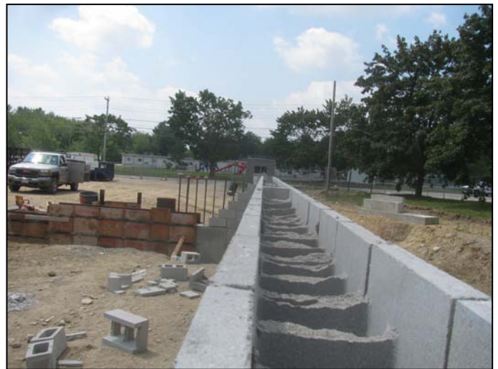
Photo 12 (4616) : Shows Nate Libby Construction Co. crew placed concrete block on the north wall of the Apparatus Bay.
