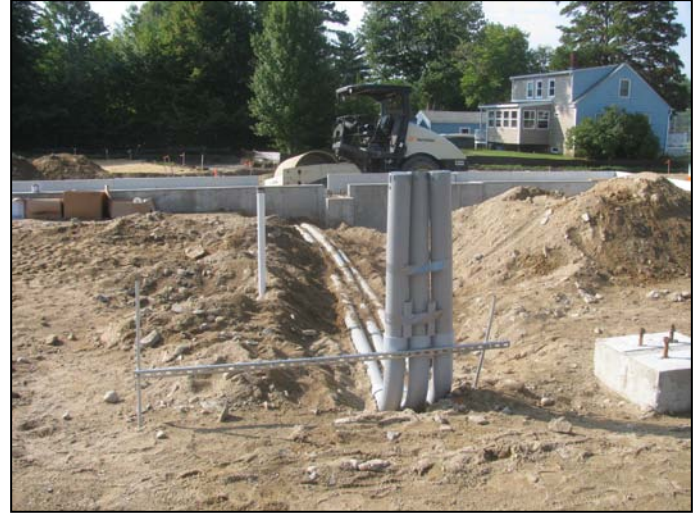
Photo 22 (4653): Shows BH Milliken Electrical Co. crew installing tele/data conduits in subgrade of the first floor slab in the Administration area.
