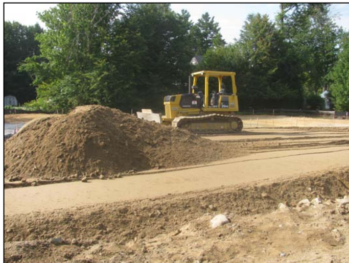
Photo 18 (4656): Shows Peters Construction Co. crew placing and compacting gravel in south access way to the rear parking lot.
