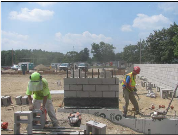
Photo 13 (4613): Shows Nate Libby Masonry Construction crew placing concrete masonry blocks on the east wall of the Apparatus Bay.
