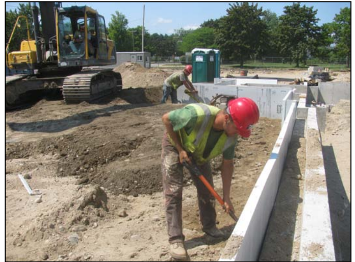
Photo 2 (4575): Shows Peters Construction Co. crew placing and compacting gravel by main entrance to fire station.
