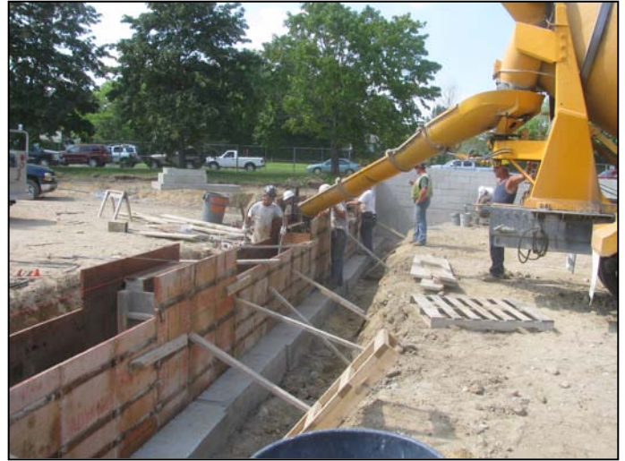
Photo 10 (4624) : Shows Lajoie Bros. Construction Co. crew placing concrete in forms for the west wall of the Apparatus Bay.
