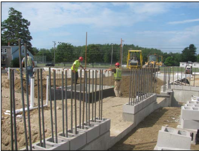
Photo 7 (4591) : Shows Nate Libby Masonry Construction crew installing concrete masonry block on "C" line wall.
