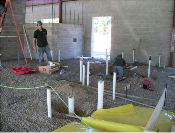
Photo 19 (0152): Shows Titan Mechanical Co. crew relocating bathroom sanitary subslab piping in the Administrative area.
