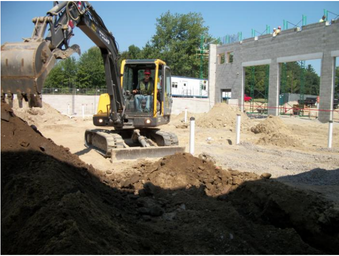
Photo 7 (0115): Shows Peters Construction Co. crew excavating trenches for sanitary piping in the Apparatus Bay.
