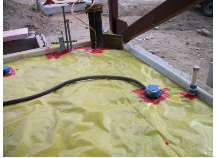
Photo 24 (0166): Shows Titan Mechanical Co. crew installed trap primers to the floor drains in the Administration area.
