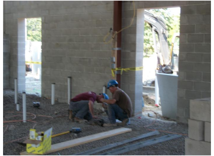
Photo 12 (0114): Shows B.H. Millekin Electric Co. crew installing ground wire and CAD welding to the ground rods in the Administration area of the Fire Station.
