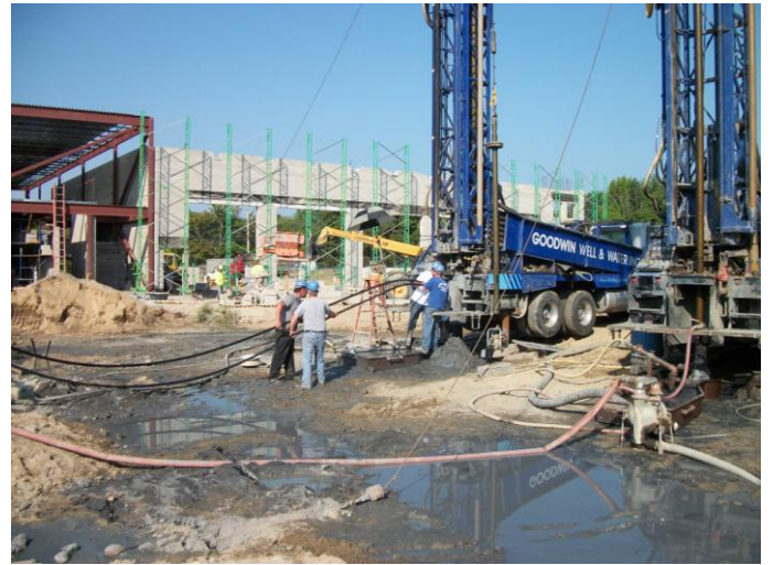
Photo 16 (0126): Shows Goodwin Well Drilling Co. crew reaming out geothermal wells No. 3 and No. 5.
