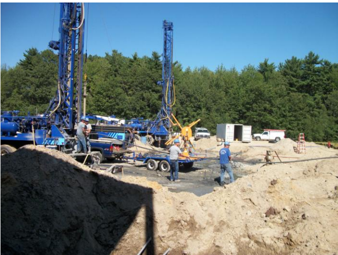
Photo 5 (0084) : Shows Goodwin Well Drilling Co. crews reaming out geothermal wells No. 2 and No. 6.
