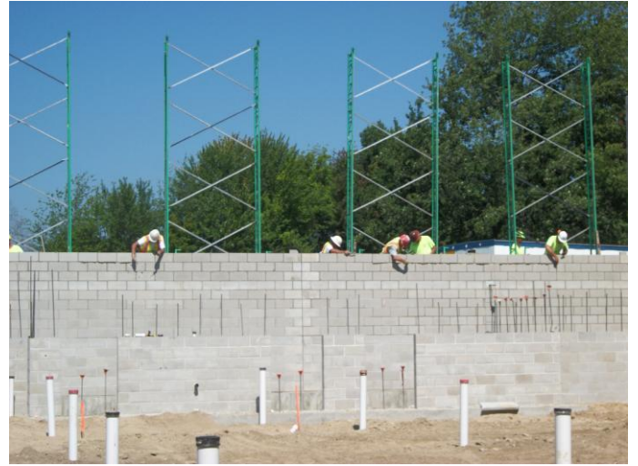
Photo 20 (0156): Shows Nate Libby Masonry Co. crew installing concrete blocks north wall of Fire Station.
