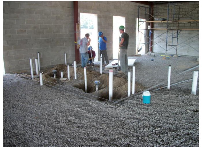
Photo 14 (0140): Shows Titan Mechanical Co. crew relocating under slab sanitary pipe in the Administration area not located correctly.
