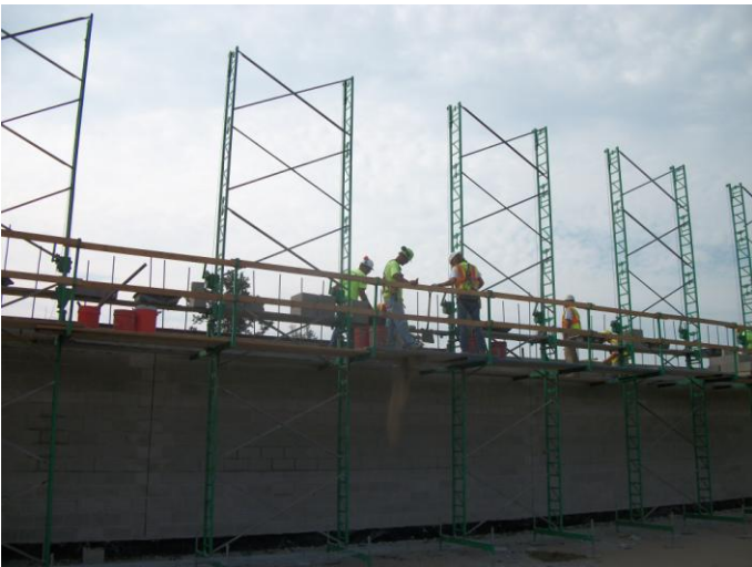
Photo 25 (0162): Shows Nate Libby Masonry Co. crew installing concrete blocks on north wall of the Fire Station.
