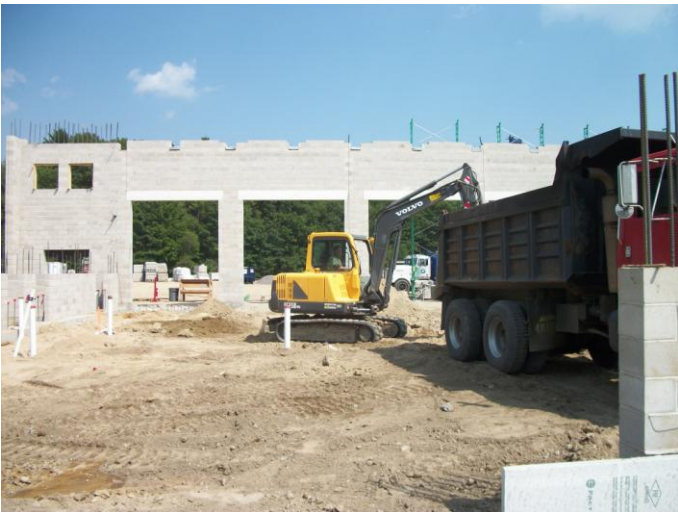
Photo 13 (0139): Shows Peters Construction Co. crew removing excess subgrade materials from the Apparatus Bay area.
