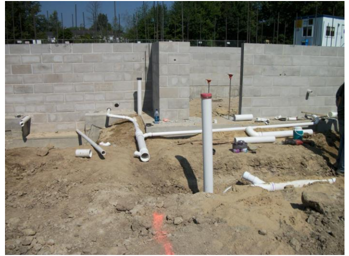
Photo 8 (110): Shows Titan Mechanical Co. crew installing sanitary piping below slab elevation in the Apparatus Bay.
