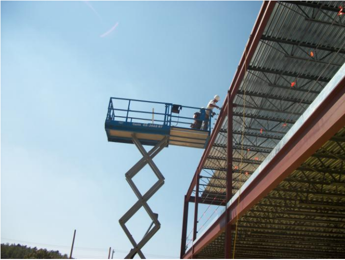
Photo 23 (0158): Shows Dirago Drywall Co. crew installing parapet framing on roof decking area of the Administration area.
