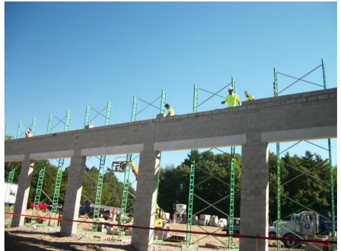
Photo 4 (0077) : Shows Nate Libby Masonry Co. crew installing concrete blocks on east wall of the Apparatus Bay.
