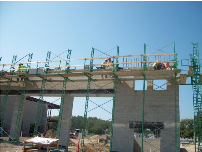
Photo 9 (0108): Shows Nate Libby Masonry Co. crew installing concrete blocks in east wall of the Apparatus Bay.
