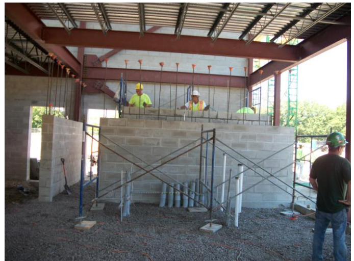
Photo 6 (0083) : Shows B.H. Millekin Electric Co. crew providing electrical conduits for installation into masonry stairwell walls.
