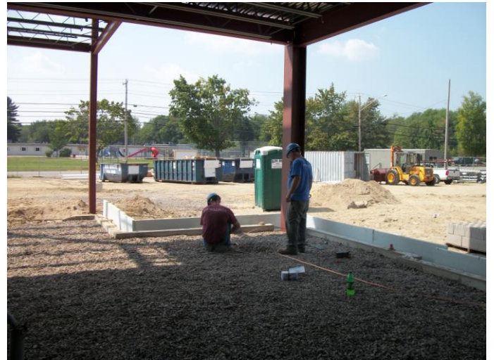
Photo 18 (0136): Shows B.H. Millekin Electric Co. crew CAD welding ground wire to ground rods in Administration area.
