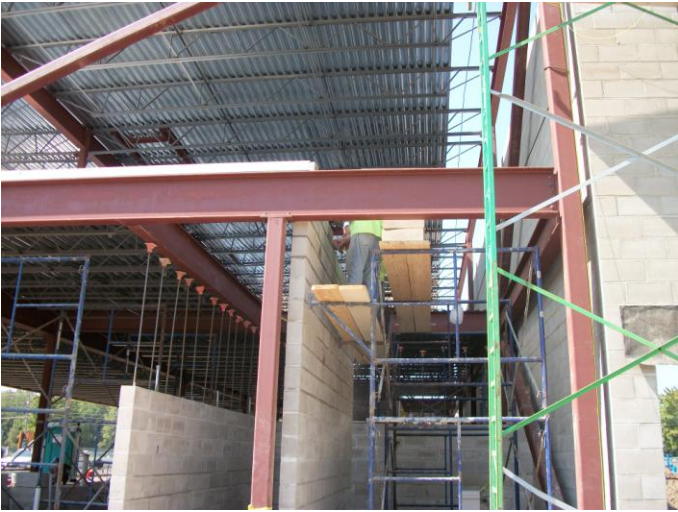
Photo 11 (0109): Shows Davis Erectors Co. crew installing decking on the second floor of the Administration area.
