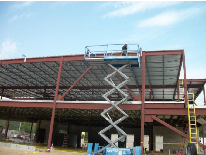
Photo 27 (0164): Shows Dirago Drywall Co. crew installing parapet framing on the roof framing in the Administration area.
