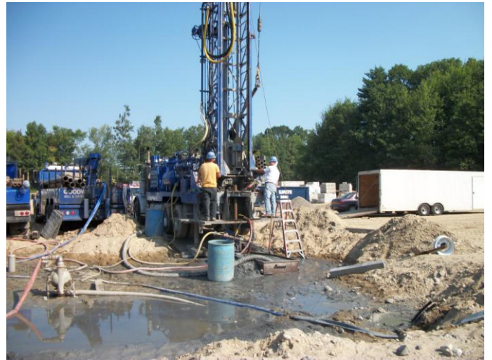
Photo 10 (0107): Shows Goodwin Well Drilling Co. crew reaming out geothermal well No. 5 and second crew setting up on well No. 3.
