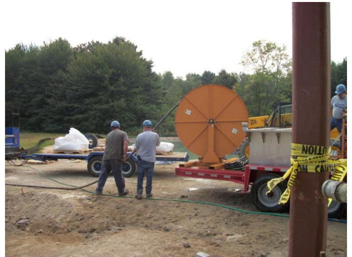
Photo 26 (0163): Shows Goodwin Well Drilling Co. crew installing geothermal piping in well No. 6.
