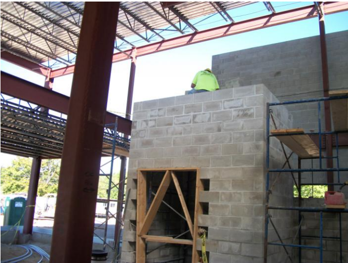
Photo 3 (0075) : Shows Nate Libby Masonry Co. crew installing masonry blocks on elevator shaft walls.
