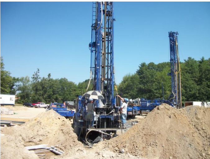
Photo 21 (0150): Shows Goodwin Well Drilling Co. crew reaming out geothermal well No. 6 and No. 1.
