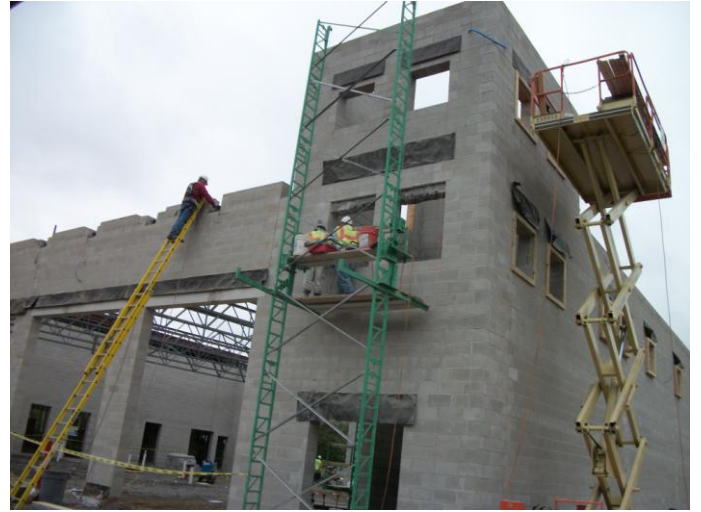
Photo 18 (0379): Shows Nate Libby Masonry Construction Co. crew demoing window openings in the training tower wall.
