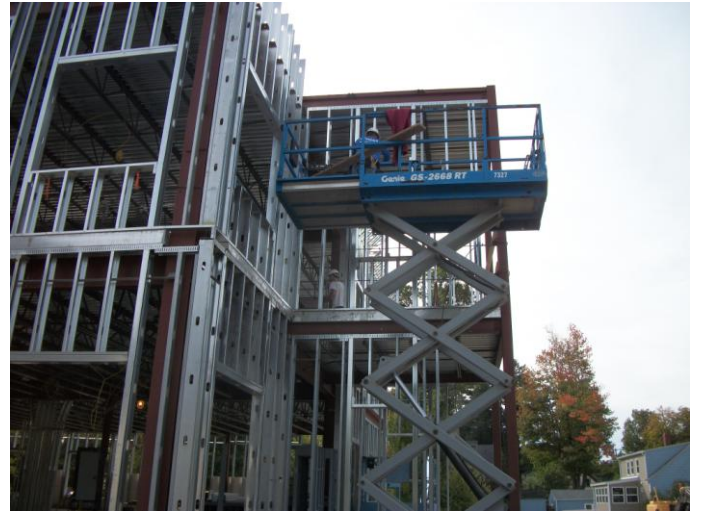
Photo 14 (0365): Shows Dirago Drywall Co. crew installing exterior wall framing 2 nd floor elevation.
