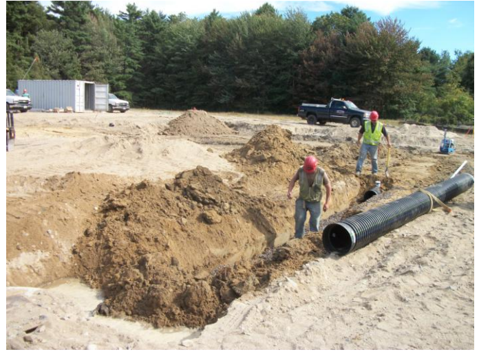
Photo 10 (0351): Shows Peters Construction Co. crew installing 12" ADA storm drain piping through the geothermal well area.
