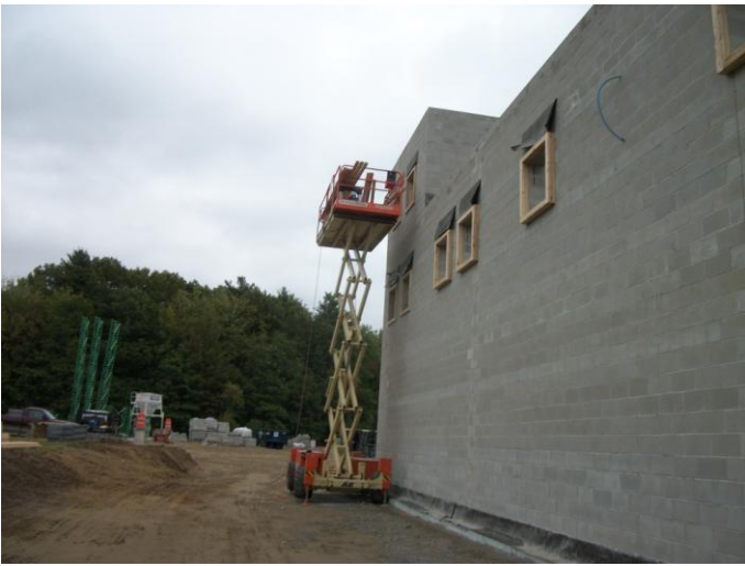
Photo 21 (0381) : Shows Pizzagalli Corp. crew installing wood blocking around the window openings north wall of the Fire Station.
