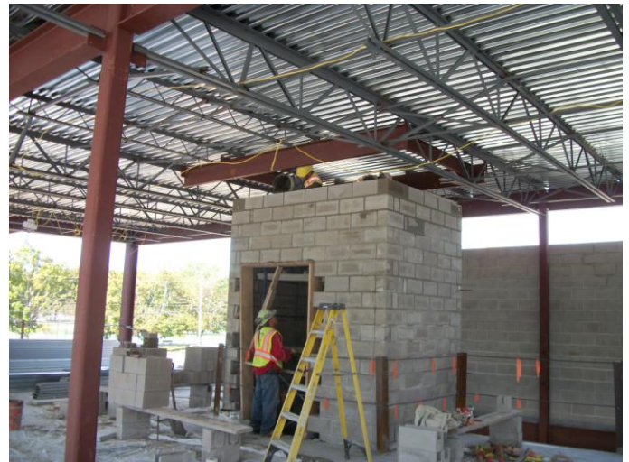
Photo 8 (0336) : Shows Nate Libby Masonry Construction Co. crew installing concrete blocks in the elevator shaft walls.
