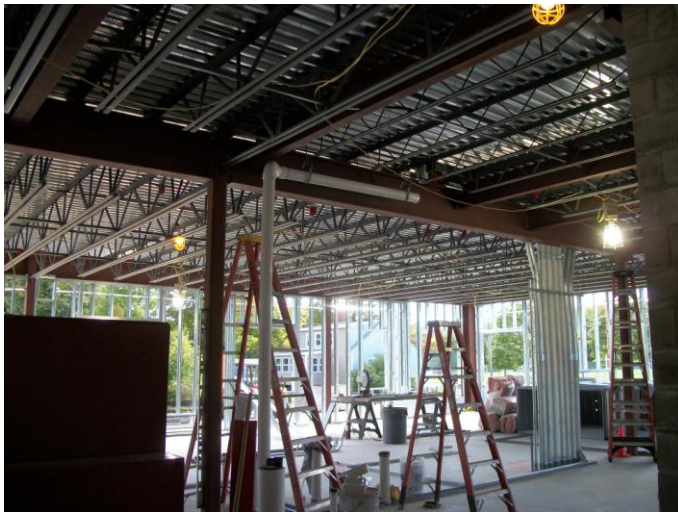
Photo 7 (0350) : Shows B.H. Milliken Electrical Co. crew installing conduits for the interior walls, 1 st floor Administration Area.
