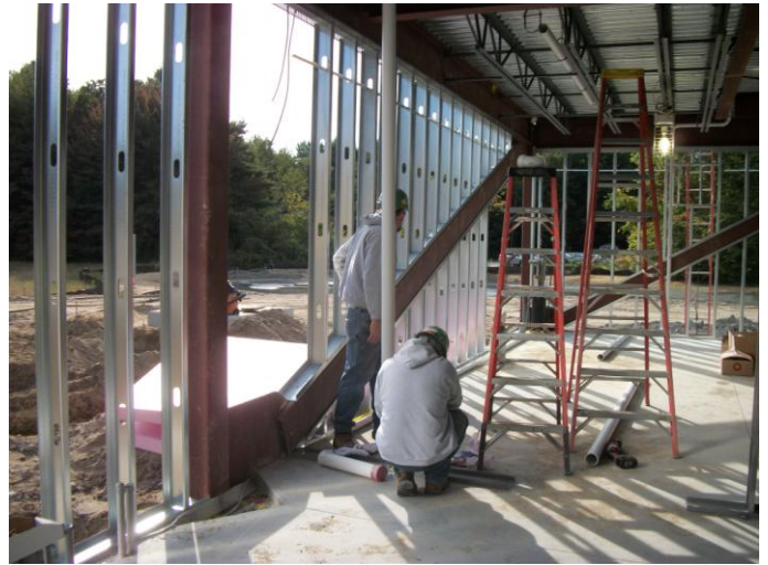
Photo 6 (0332) : Shows Titan Mechanical Co. crew installing vent piping in mechanical room, 1 st floor Administration Area.
