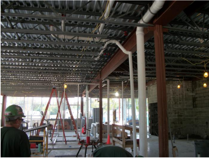
Photo 17 (0395): Shows B.H. Milliken Electrical Co. crew installing conduits to 2 nd floor elevation.
