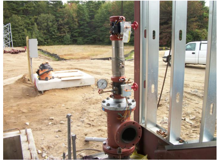
Photo 16 (0387): Shows Titan Mechanical Co. crew has installed the sprinkler system control valve in the mechanical room.
