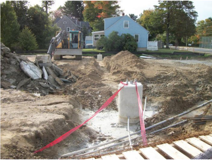
Photo 13 (0364): Shows B.H. Milliken Electrical Co. crew has installed electrical conduits to the sign area and the light pole bases.
