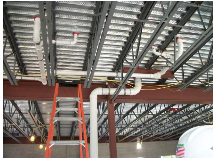
Photo 12 (0367): Shows Titan Mechanical Co. crew installing sanitary and vent piping in 1 st floor elevation Administration Area.
