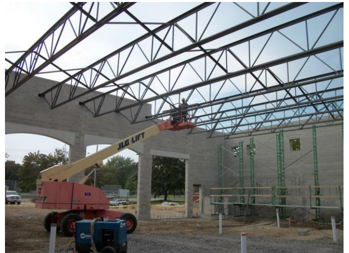
Photo 20 (0401): Shows Davis Erector Co. crew installing structural bar joists in the roof of the Apparatus Bay.
