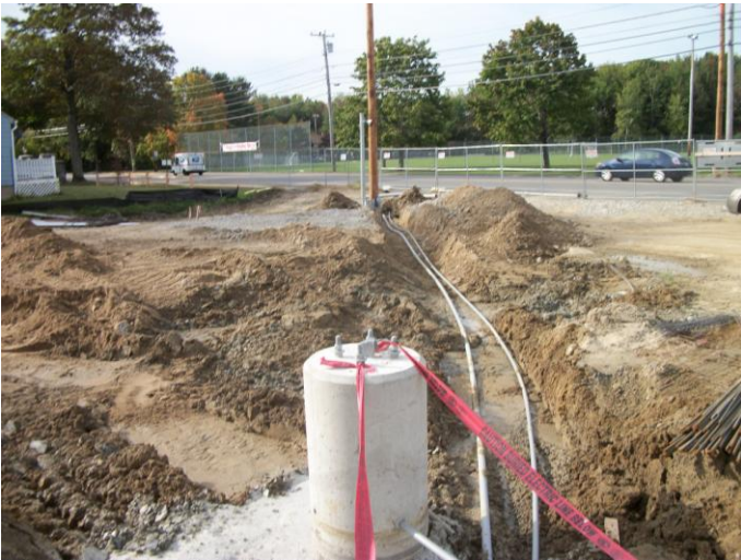
Photo 11 (0363): Peters Construction Co. crew has excavated for the electrical conduits to the light pole bases.
