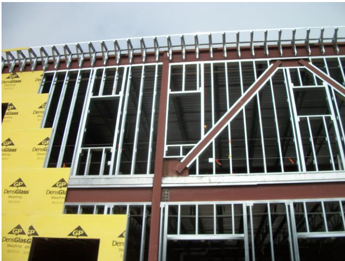
Photo 19 (0389): Shows Dirago Drywall Co. crew installing DensGlass sheathing on the south wall of the Administration Area.
