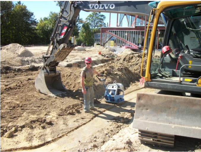
Photo 5 (0347) : Shows Peters Construction Co. crew backfilling and compacting material over the geothermal well piping.
