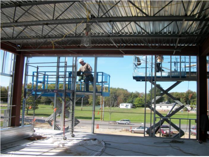
Photo 9 (0337): Shows Dirago Drywall Co. crew installing exterior wall framing west wall of the entrance area.
