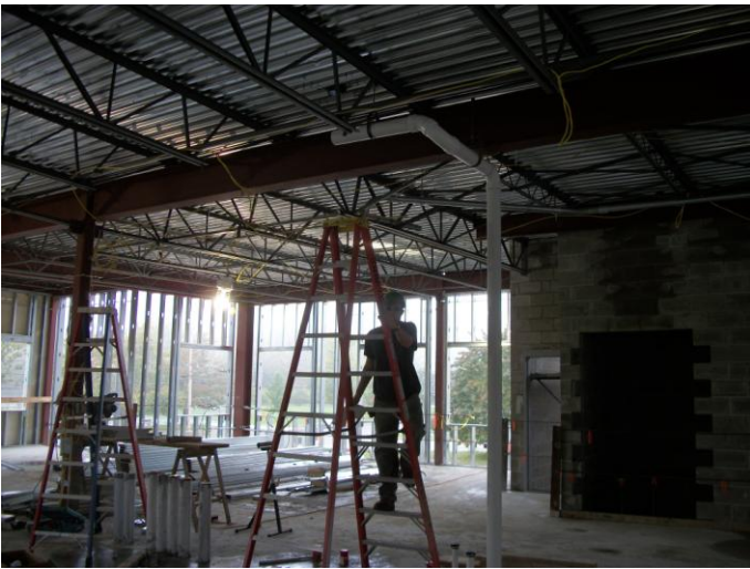
Photo 15 (0474) : Shows Titan Mechanical Co. crew installing roof drain piping, 2 nd floor elevation in the Administration Area.
