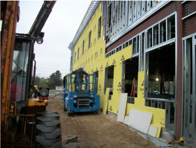
Photo 1 (0410): Shows Dirago Drywall Co. crew installing dens glass sheeting on the south wall of the Administration Area of the Fire Station.
