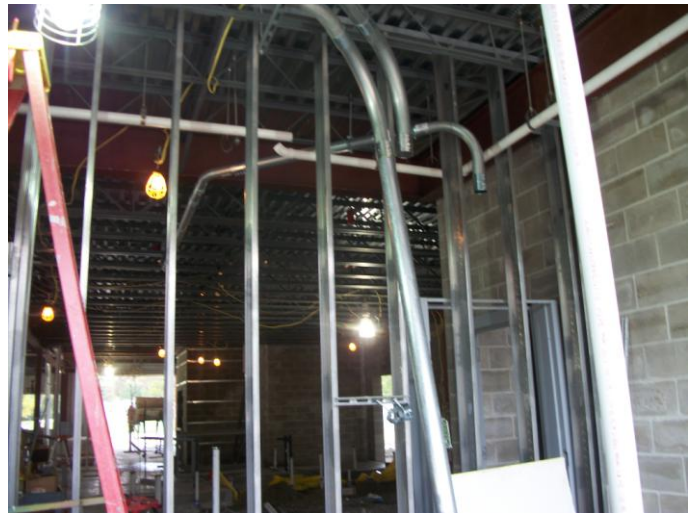
Photo 16 (0479) : Shows B.H. Milliken Electrical Co. crew has installed electrical conduit in the overhead to the electrical room.
