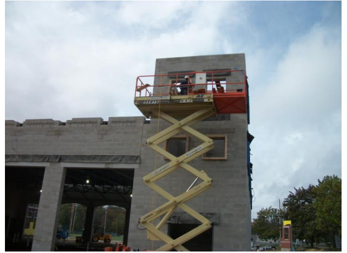
Photo 18 (0478): Shows Pizzagalli Corp. crew installing blocking around window openings in the training tower wall.
