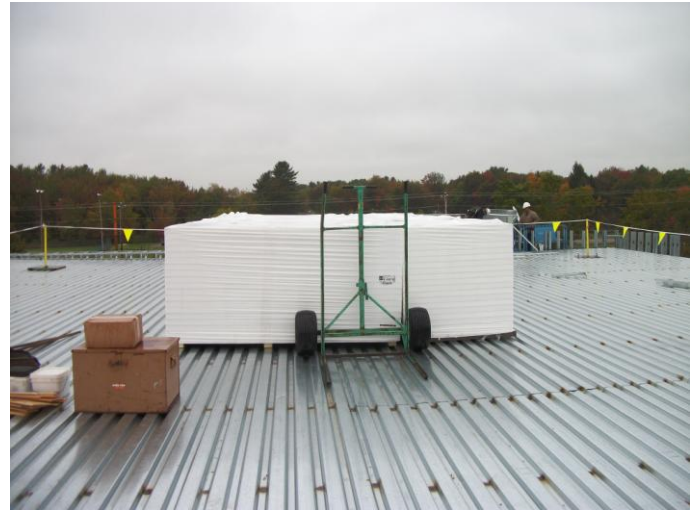
Photo 2 (0415): Shows SMR Roofing Co. crew stockpiling roofing supplies on the roof of the Administration Area.
