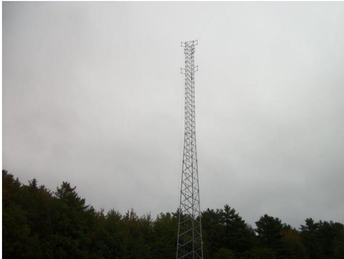
Photo 7 (0433): Shows Green Mountain Communication Co. crew has completed the erection of the communication tower.
