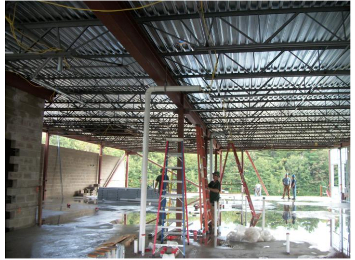
Photo 10 (0455) : Shows Titan Mechanical Co. crew installing rain leader piping for the roof drains on the 2 nd floor elevation of the Administration Area.
