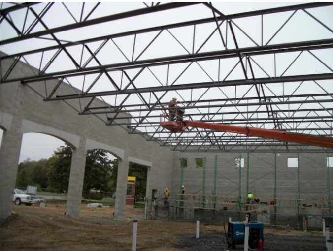
Photo 3 (0404): Shows Davis Erectors Co. crew installing bracing on the roof joists in the Apparatus Bay.
