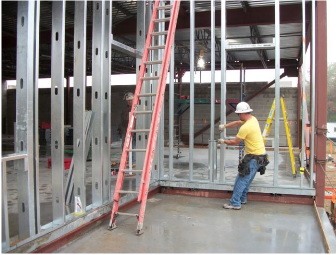
Photo 17 (0473): Shows Dirago Drywall Co. crew installing exterior wall framing in the patio area.
