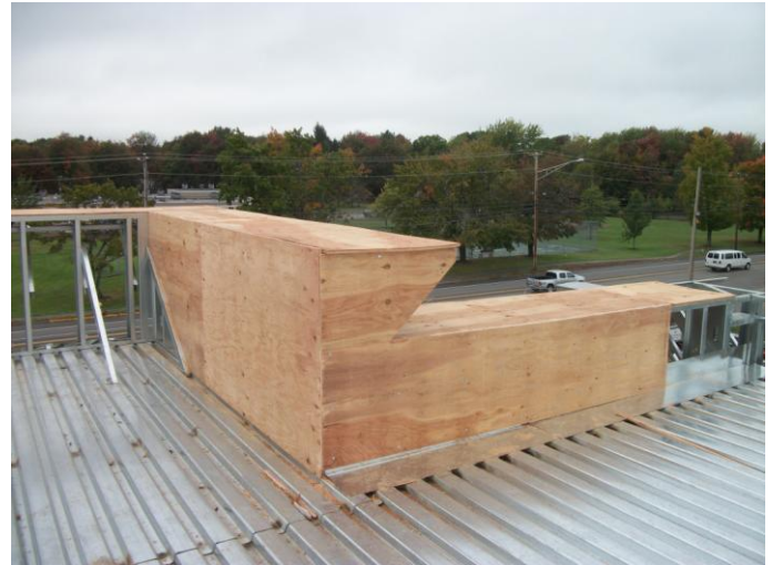
Photo 8 (0441): Shows SMR Roofing Co. crew has installed plywood to the parapet framing on the west end of the roof of the Administration Area.
