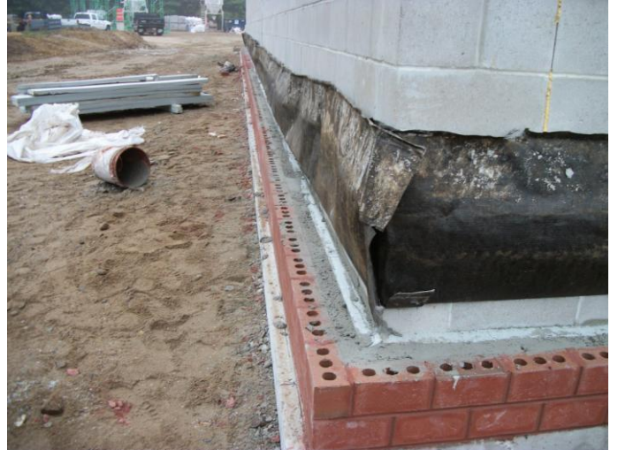
Photo 14 (0468) : Shows Nate Libby Construction Co. crew has installed insulation and grout inside of the brick veneer at the foundation elevation.
