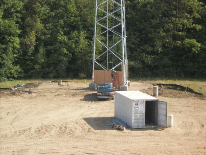
Photo 13 (0460) : Shows Pizzagalli Corp. crew enclosing the base of the communication tower to limit access for safety.
