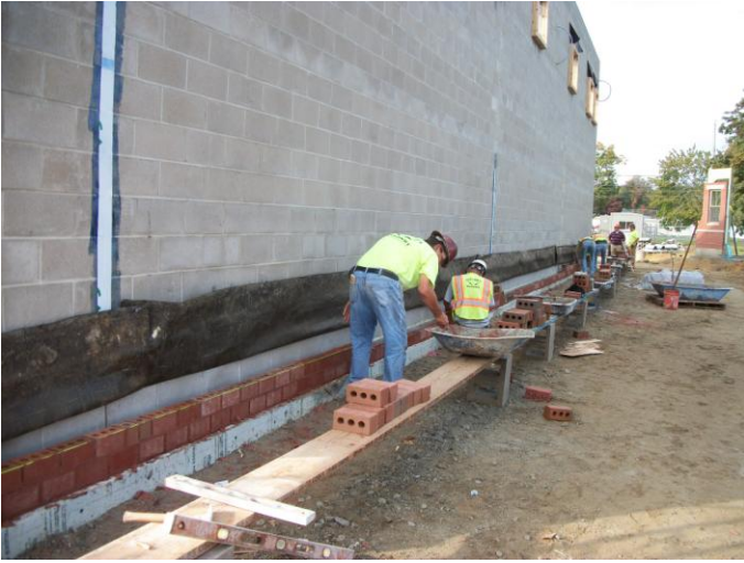
Photo 9 (0450) : Shows Nate Libby Masonry Construction Co. crew installing brick veneer on the north wall of the Fire Station building.
