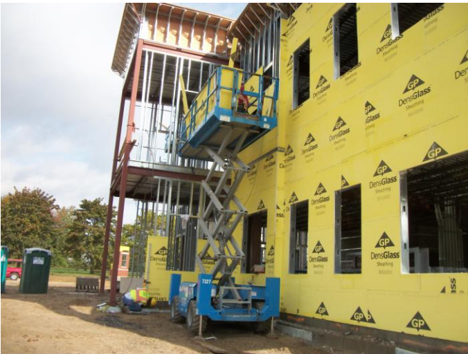
Photo 11 (0453) : Shows Dirago Drywall Co. crew installing dens glass sheeting on the west wall of the Administration Area.
