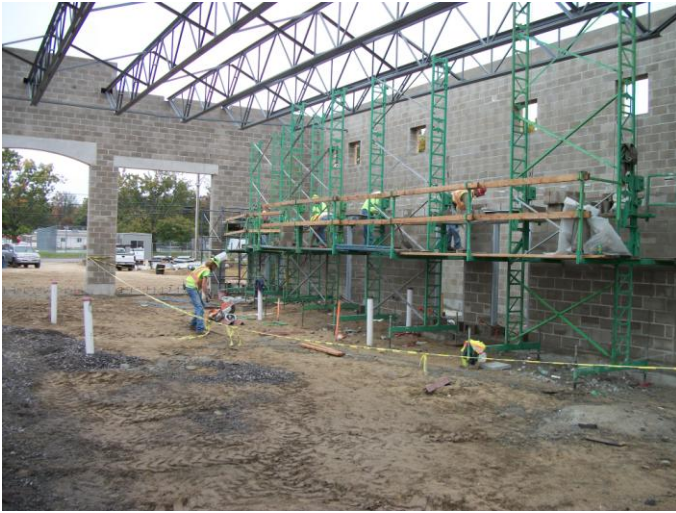
Photo 5 (0434): Shows Nate Libby Masonry Construction Co. crew installing concrete block on mezzanine wall.
